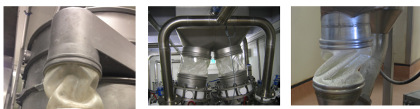
Installation gap too small
